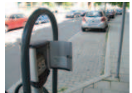
Electric car charging points
